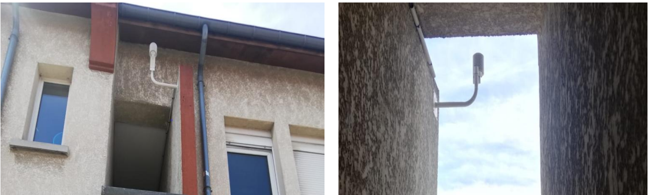
Figure 16: Exterior sensors installed on the façade of the building.
