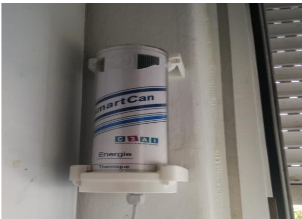
Figure 17: Connectors sensors of energy consumption.
