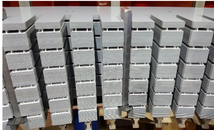
Figure I.3. Stator core of the Hydro generator La Coche - G5 (237,8 MW) during the assembly step (Image from EDF).
