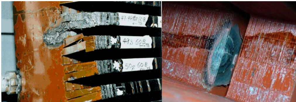
Figure I.9. Degradation of stator core due to a short-circuit between the stator laminations. [4]
