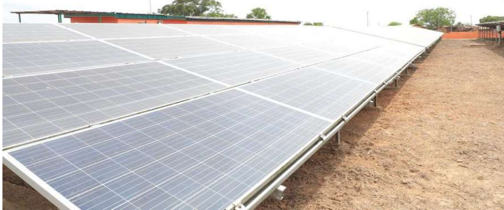
Figure 32. Minicentrale hybride de Dybikro (Source : CI-Energies)
