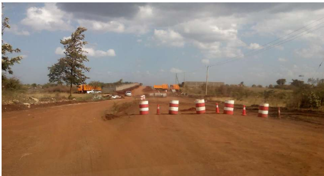
Figure 4.20: A diversion during the construction of the Ruiru to Uplands road on 13 December 2018
