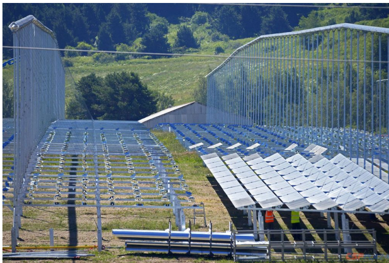
Figure 1.3: eLLO 9 MW linear Fresnel CSP plant (Llo, France).
