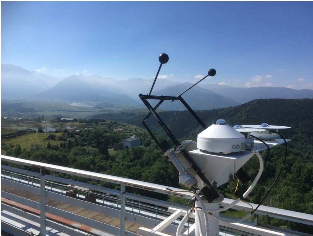
Figure 2.4: Pyrheliometer installed on a solar tracker at the PROMES laboratory (Odeillo, France).
