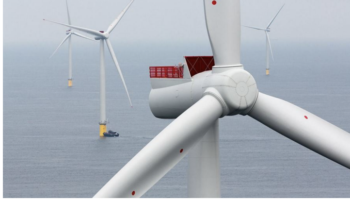
Figure 5.5: Picture of several SWT-6.0-154 gathered in an offshore wind farm, taken from Siemens Gamesa Renewable Energy website .
