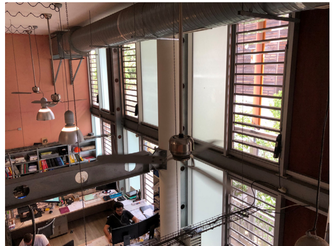
Fig. 2. View of the louvers and ceiling fans in open-spaces.
