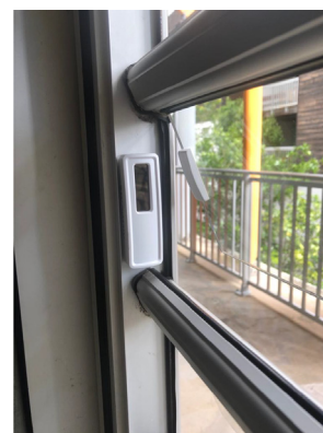
Fig. 3. Opened window (called louvers) with magnetic contact.
