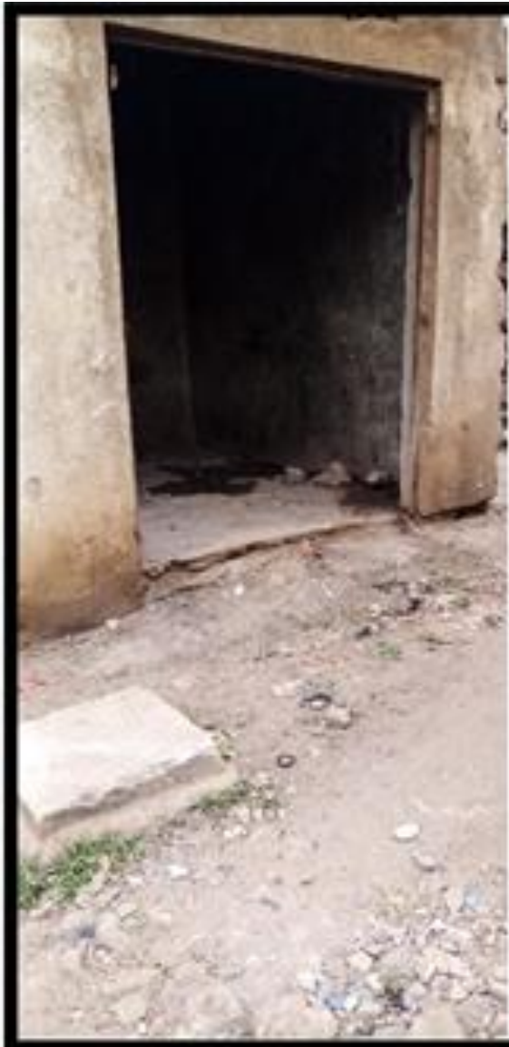
Stall A (empty vandalized stall)
