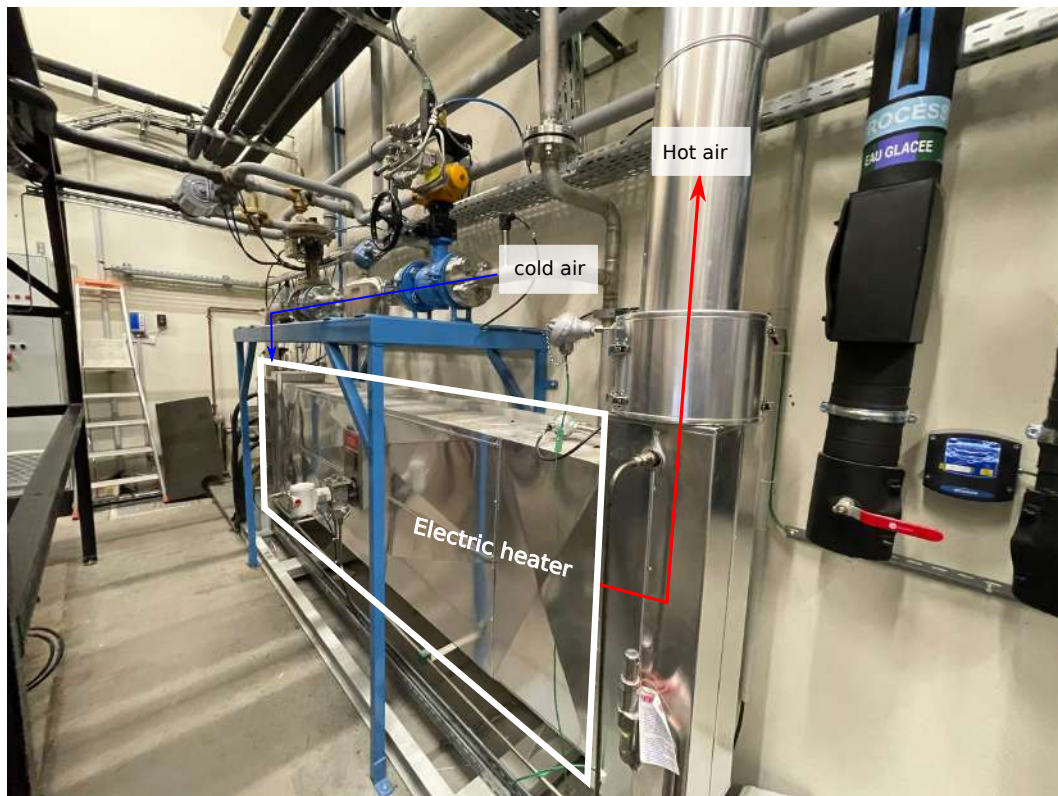
Figure 5.5: Picture of the electric heater system.
