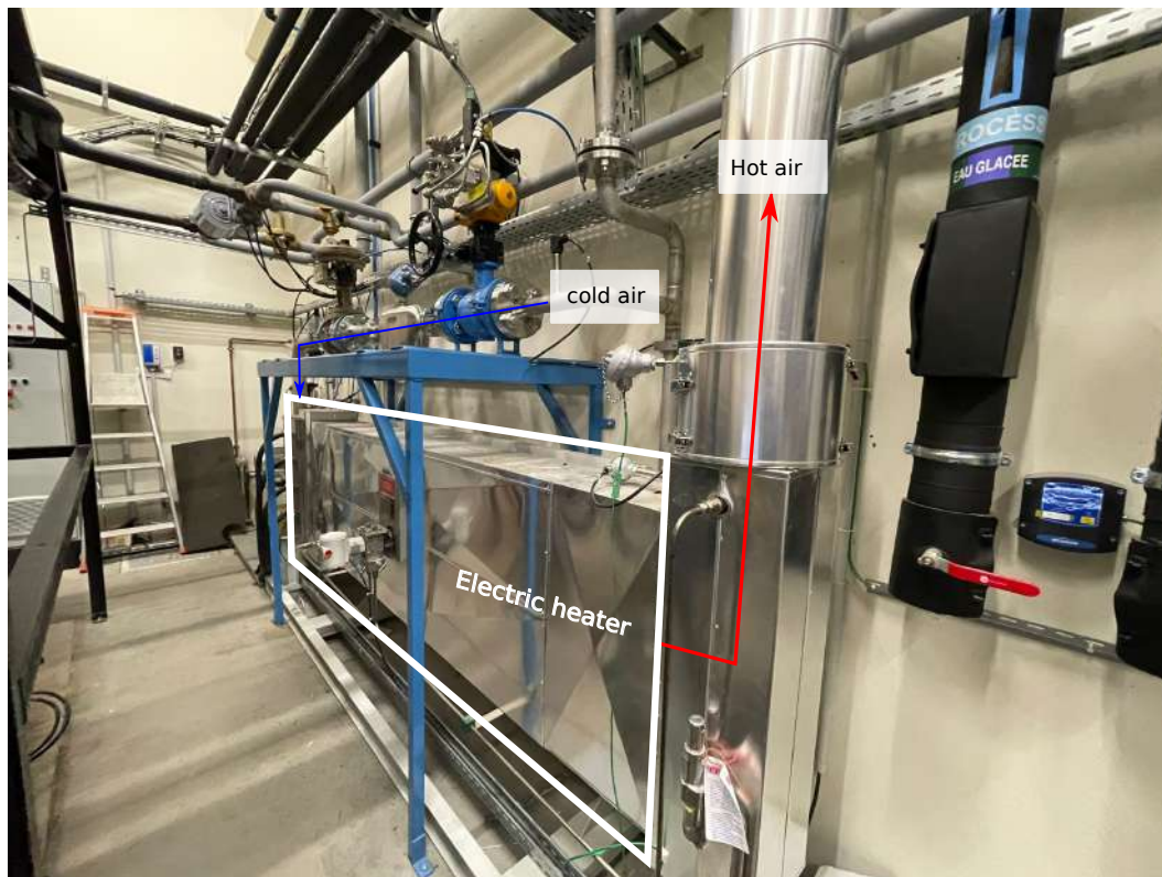
Figure 5.5: Picture of the electric heater system.
