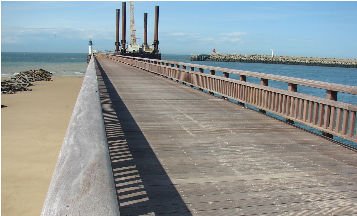
Figure 94: Use of ekki on the deck of Calais West pier. Credit: Marc Igigabel, Cerema.
