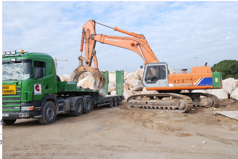
Figure 93: The loading of a piece of armourstone in the port of Marseille. Credit: Grand Port Maritime de Marseille.
