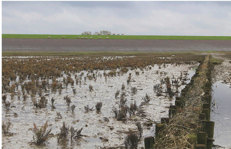
FIGURE 12 | Brushwood dams in the Dutch Wadden Sea, which create artificial shelter for salt marsh vegetation from waves and currents. The levee is visible in the background (Photo: V. Vuik).
