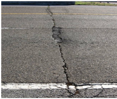
A – Fissure transversale
