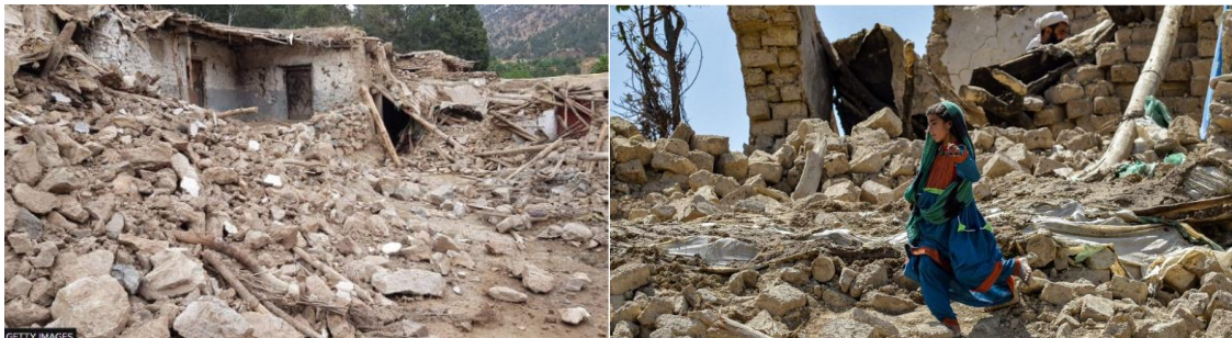
Figure 16: Earthquake damage to earthen houses in Paktika, Afghanistan (BBC, 2022)
