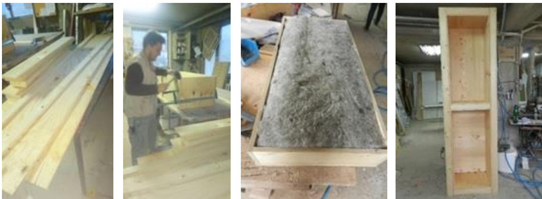
Figure 66. Pictures during the production of the GDC wall prototype. From left to right: 1.all parts cut to measure, 2. Making wooden wall structure, 3. wooden box filled with natural sheep wool, 4. Wooden wall structure. (photo Androšević)
