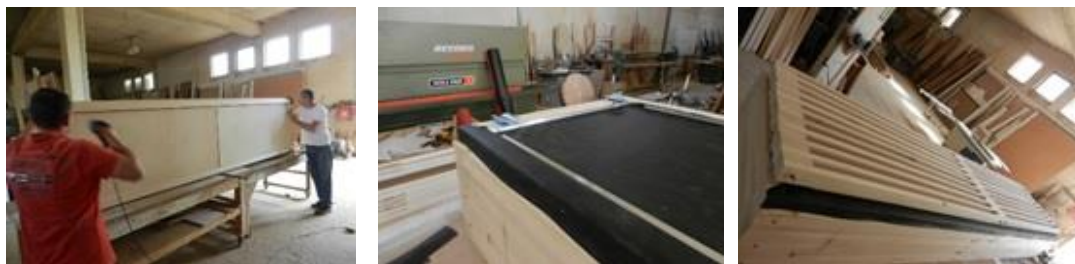
Figure 71. Pictures of the GDC wall prototype made in Herzegovina. Picture left – inserting wooden boxes in the wooden frame, middle – fixing water vapor permeable membrane with Alu L shaped profile and right – wall prototype finished. (photo Androšević)
