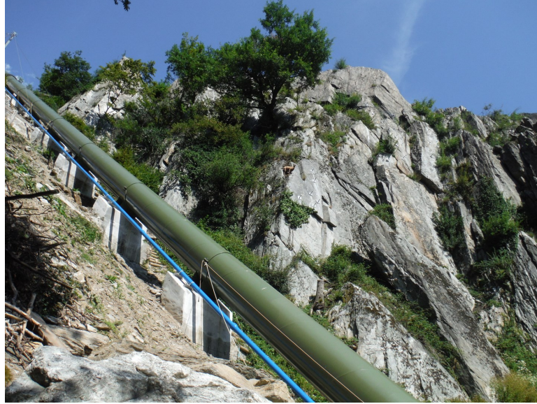
FIGURE 3.1: Example of a penstock operated by EDF.
