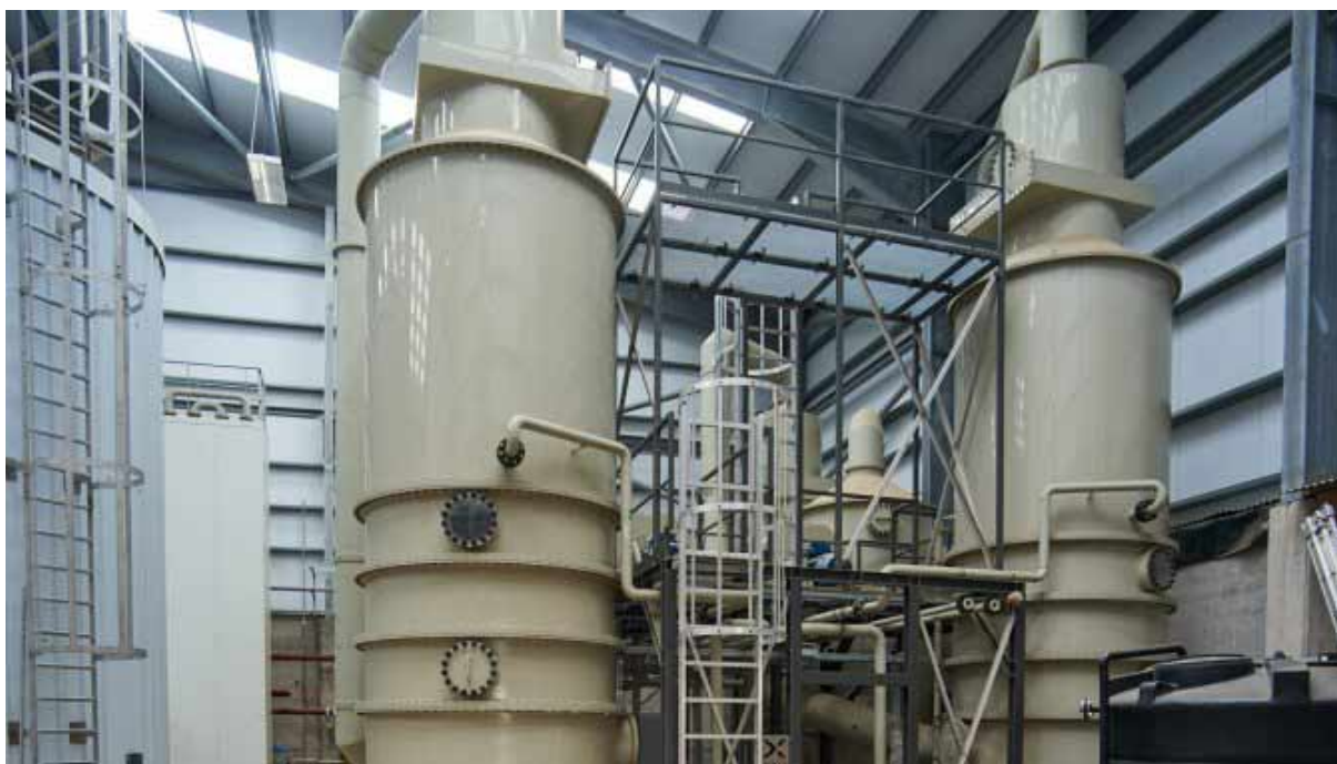
Figure 15: Nix® technology (Xergi) integrated in full-scale plant – picture from (Xergi, website)
