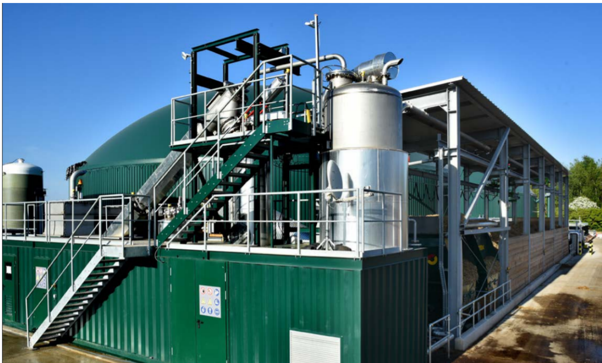
Figure 14: Economizer SE in a UK biogas plant built by Future Biogas Ltd – picture from (Future biogas Systems, website)
