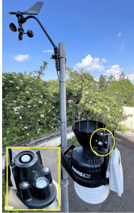
Figure 7-13: The installed weather station. The solar pyranometer is marked with yellow and zoomed.
