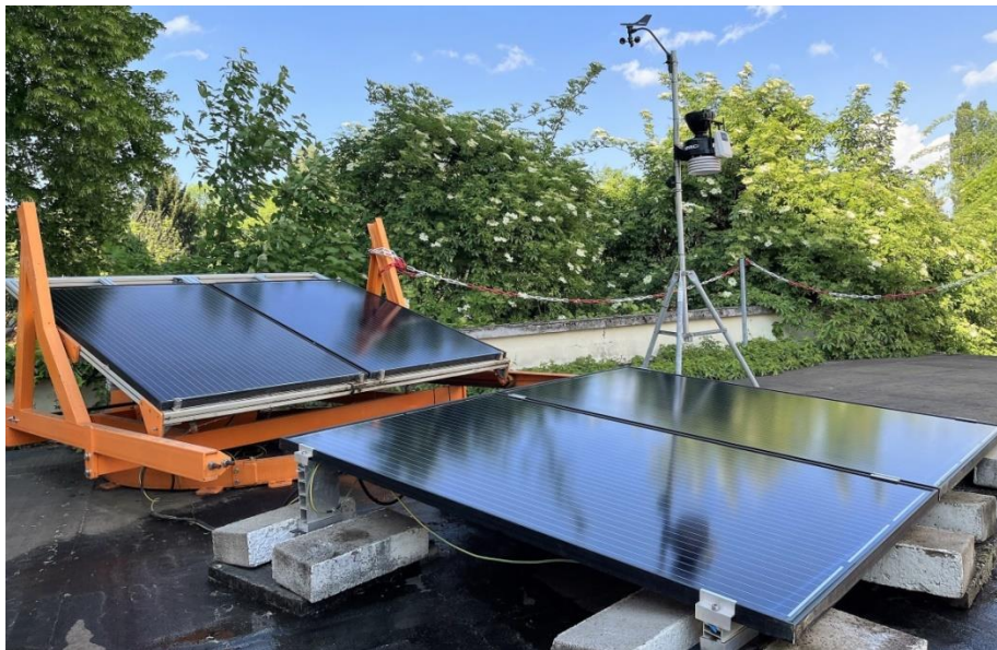
Figure 7-9: The installed PV panels at INSA ICUBE laboratory.
