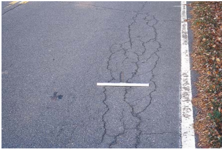
Figure 2.3: Example of fatigue cracks on pavement [21].
