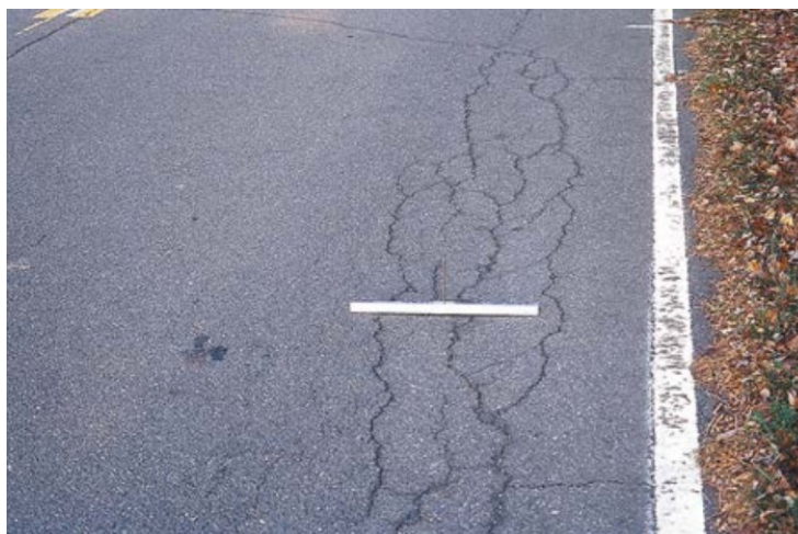
Figure 2.3: Example of fatigue cracks on pavement [21].
