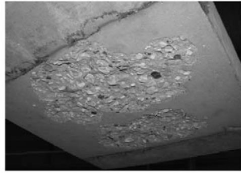
(b) Exposed surface of slabs after fire test (Mindeguia et al. [55])
