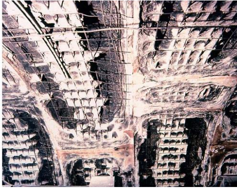
(a) Fire damage to concrete of Channel Tunnel indicating severe spalling
