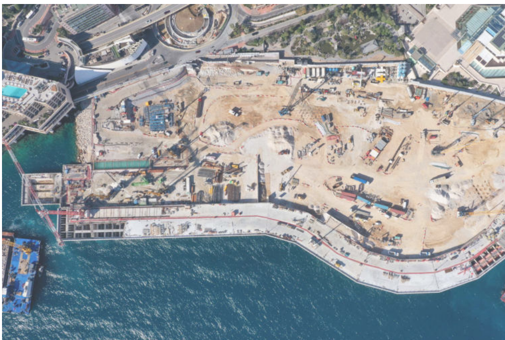
Fig. 22 - Land reclamation along the urban amphibious of the city of Monaco, in the homonymous principality. The operation is intended to gain about 61,000 square meters of coastal land from the Mediterranean sea (source: www.newcivilengineer.com ).
