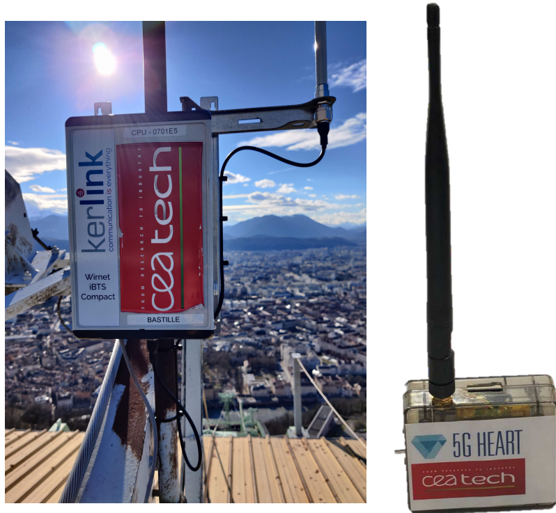
(a) Gateway BS_3 which is installed on the roof near the cable car station at Bastille, (b) Tag which was used to collect the data in Grenoble
