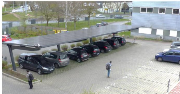
Figure 34: PV parking shade installation for nine spots.
