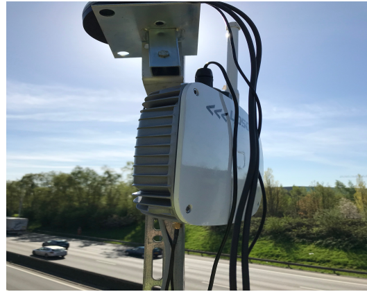
(b) Installed RSU on the Highway
