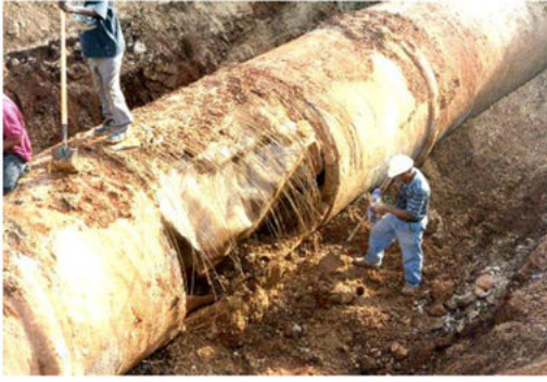
(a) Collapsing of a water supply pipe in Puerto Rico, source [Abuiziah et al., 2013]
