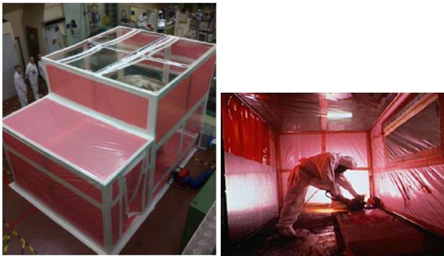
Figure 1-3 Airlock with flexible walls (left) and dismantling operations inside an intervention airlock (right)
