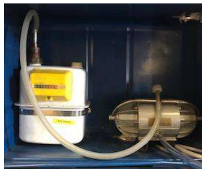
Figure 3-19 A volumetric flowmeter connected to a piston pump
