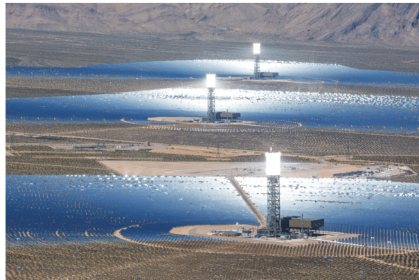
Figure 3 – The Ivanpah Solar Electric Generating System [41]
