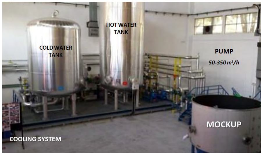
Fig.3.1 - Overview of PLATEAU facility
