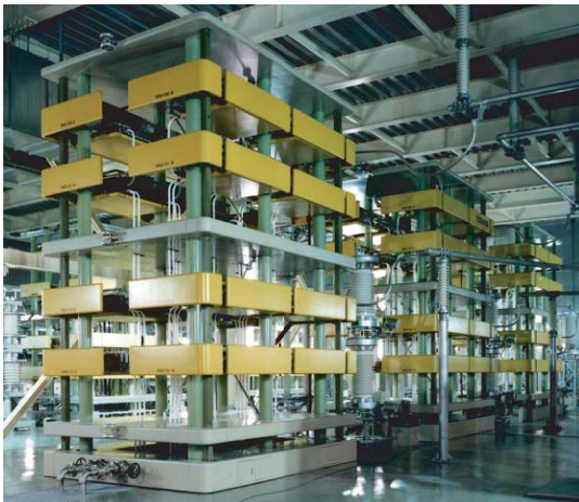
Figure I-4: thyristor tower for the frequency converter on Shin-Shinano side
