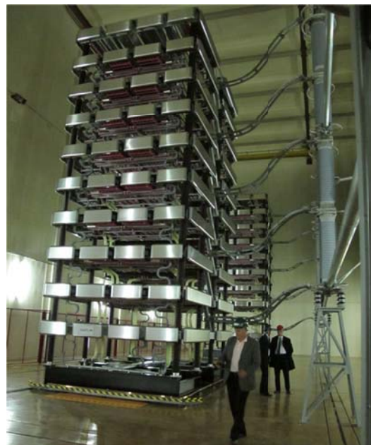
Figure I-5: Thyristor tower of the France-England connection on the french side
