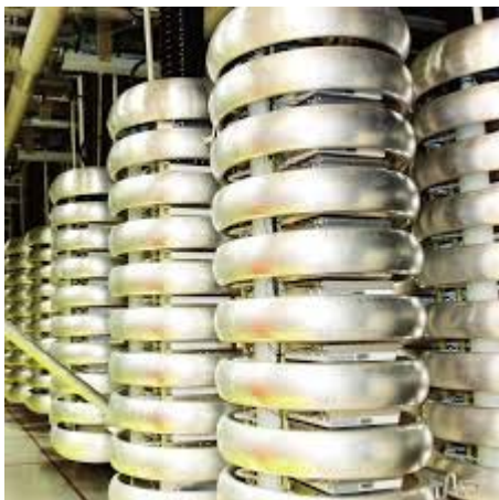
Figure I-7: Typical series valve tower of ABB
