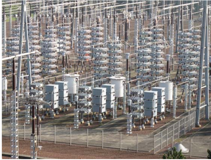
Figure I-42: LC shunt filters at « Les Madarins » converter station in France - England Interconnection
