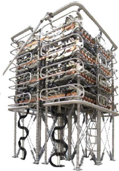
Figure I-10: typical MMC tower of a phase based on IGBT and proposed by SIEMENS
