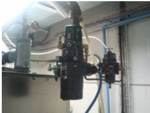
Figure 3.6: Photograph of the pressure regulation pneumatic valve.
