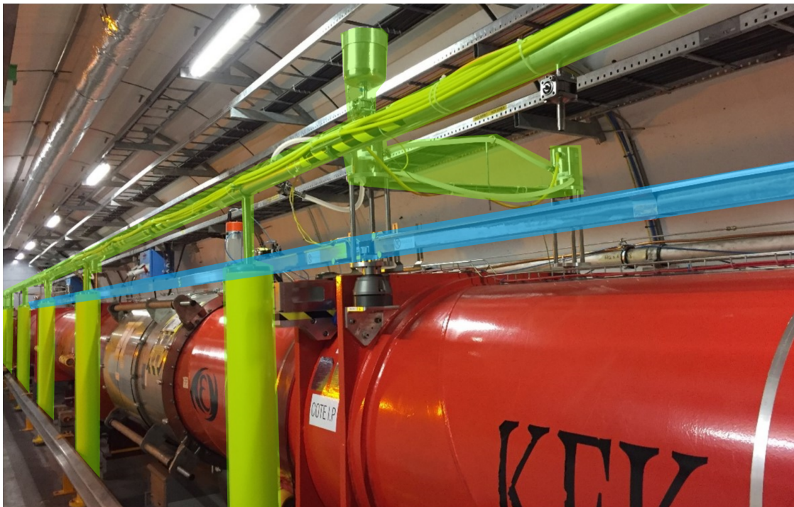
Figure 2.8: Picture of the installation in the tunnel near the experiment. The HLS infrastructure has been highlighted in light green: stable support pillars, water network, sensors and soft connection pipes. The WPS infrastructure has been highlighted in light blue: sensor, wire and wire protection.
