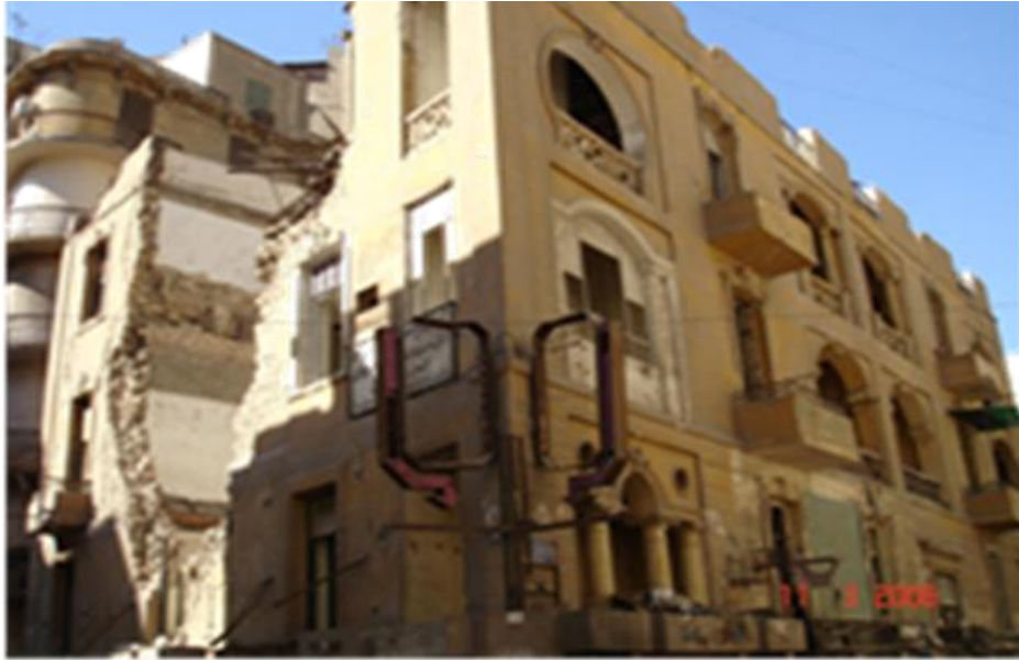
Figure 33: Deliberate destruction by constant bulldozing for delisting (Building no10, El-Bostan Street). Source: (NOUH guidelines, 2009)
