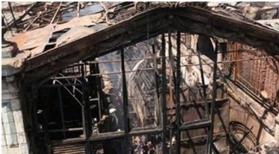
Figure 30: Attaba Market after devastating fire. Source: (Ahrām online, 2019)
