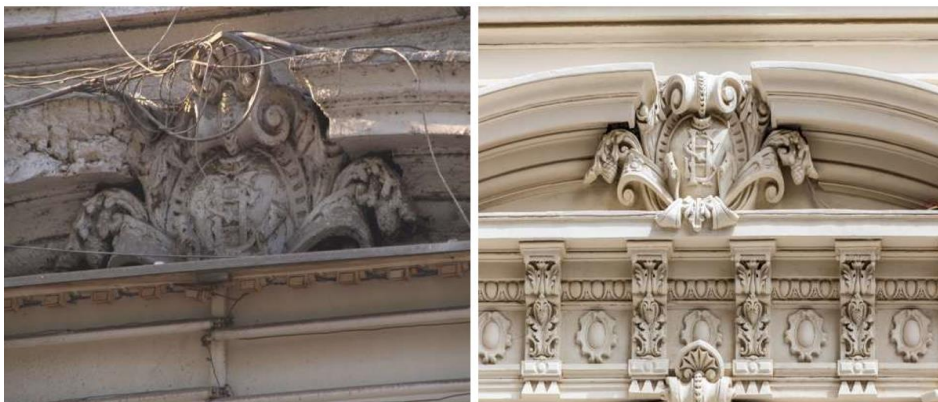
Figure 64: The state of the decorative elements before and after restoration work. Source: Al- Ismailia Company
