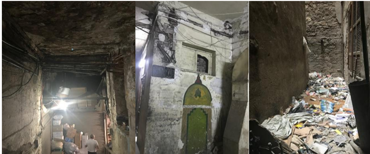
Figure 32: The deterioration due to the lack of maintenance and infringement inside of khedival Cairo building. Taken by the author, 2019.
