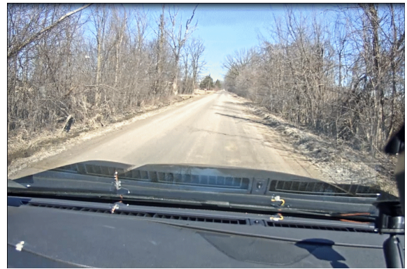
(c) Damaged road
