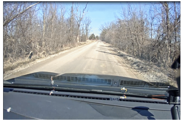
(c) Damaged road
