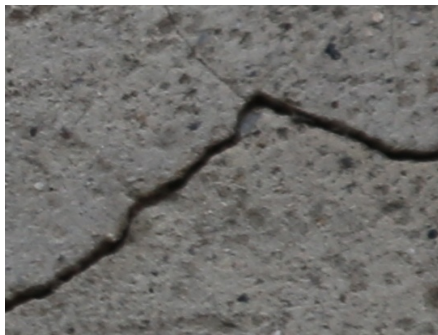
(a) Fissure (source : [25])
