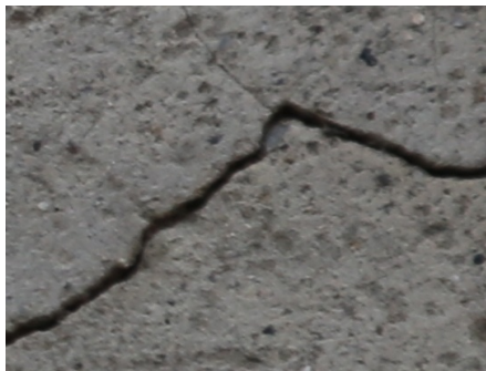
(a) Fissure (source : [25])
