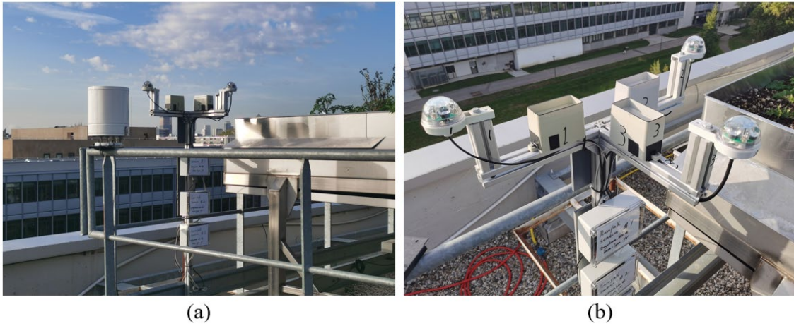
Figure 5-16. Recent rainfall monitoring station installation: (a) Panorama, (b) Top view.
