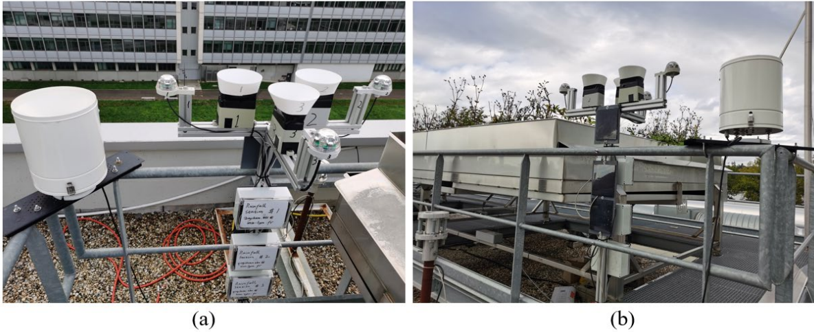
Figure 5-17. Last rainfall monitoring station installation: (a) After increase of the funnel area, (b) Back view showing the three solar panels for three rainfall monitoring stations.
