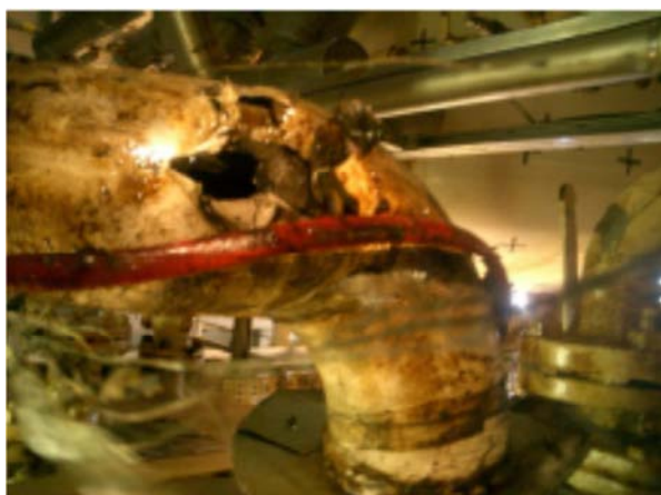
Fig. IV.4. Example of MIC-related failure; Punctured pipe, Valhall 2009.
