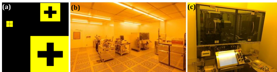
Figure A-8 (a) Image of Alignment cross on the side of the mask in 2-D design file, (b) 58 m 2 area in class 100 dedicated to photolithography and substrate sealing, (c) Automatic alignment equipment in ESIEE Paris CLEANROOM [283]
