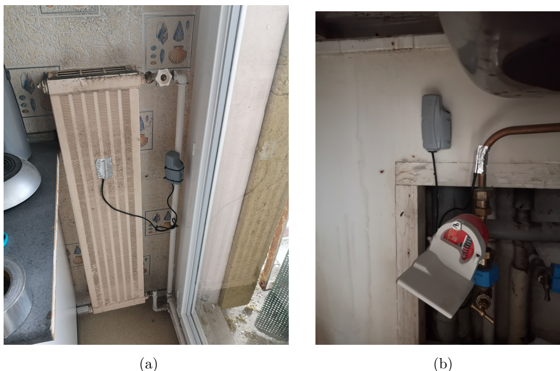
Figure 2.6: Installation of temperature sensor for DHW (a) and a heater (b) in apartments.
