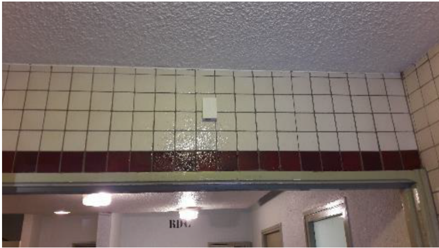
Figure 2.9: Infrared presence sensor in buildings shared areas.
