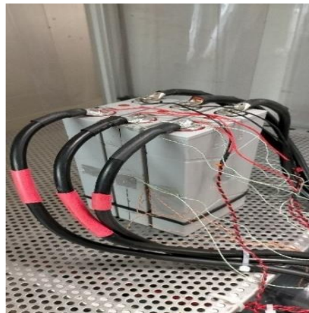
Figure IV.16 Tested 60Ah Li-ion battery pack.
