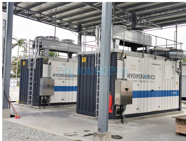
Figure 1.2: Two electrolyzers are used to produce hydrogen via electrolysis (The Borneo Post, 2020)
