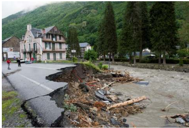
FIGURE 1.1: Infrastructural damages caused by the Garona river flash flood of 2013, June 18 th , in Les (Spain). (©AEAG P. Barthe)
