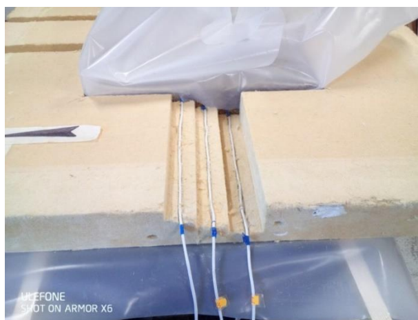
Figure 4.7. Sensor installation within the tested wall
