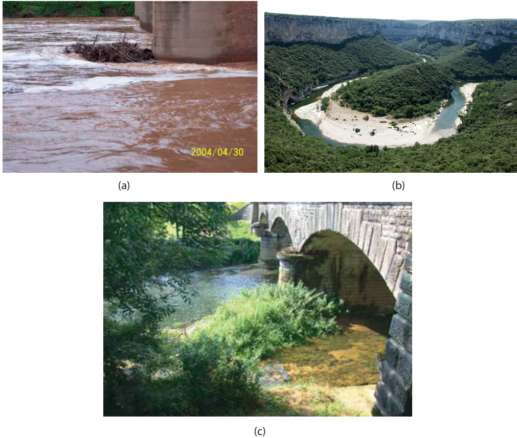
Figure 2.7: Photos of damages on river channel: (a) debris; (b) bars (sediment deposition); (c) excessive vegetation.
