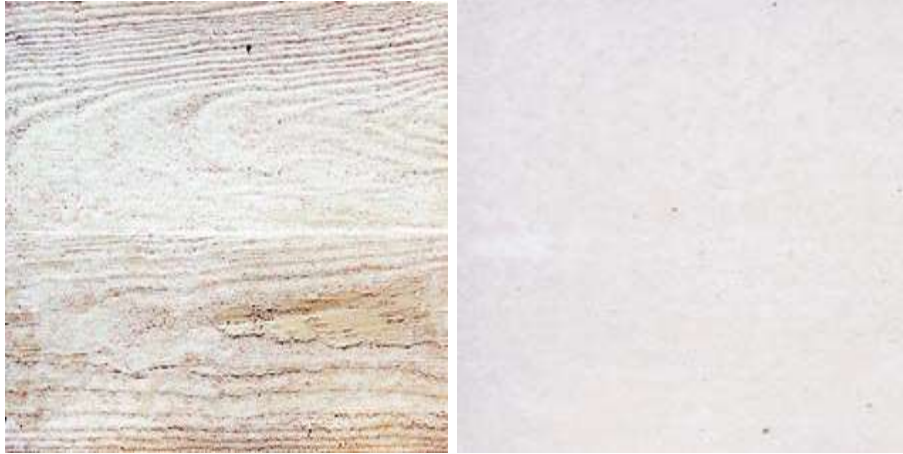
Figure 31 Two surfaces made with an identical concrete composition and casting procedure, but different formwork [126]
