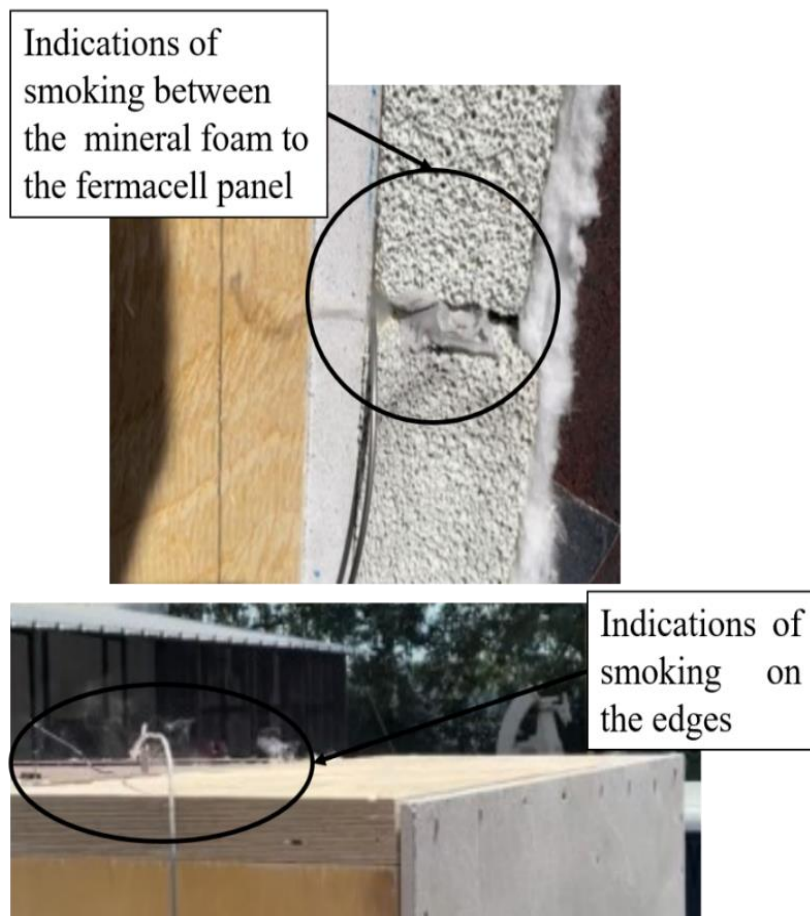
Figure 8.6: Smoking indications on edges of the exposed face of the wall
