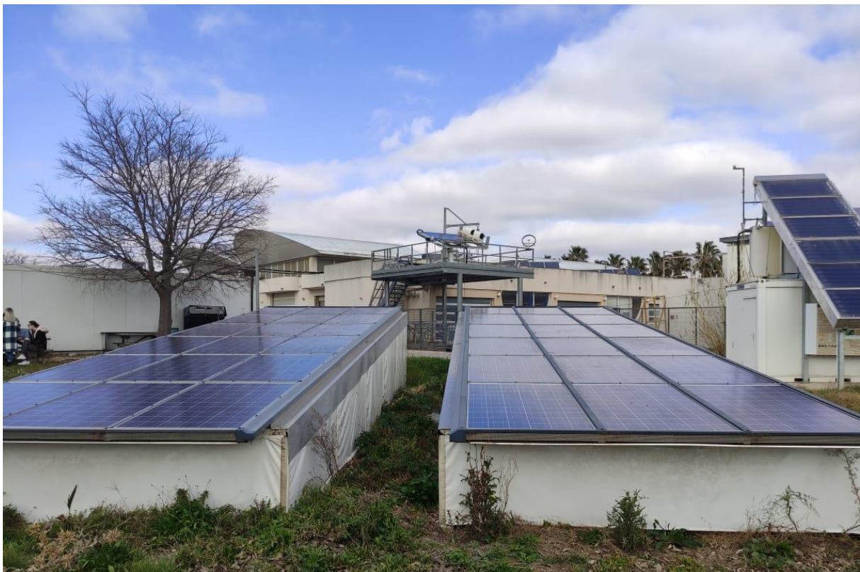
Figure 3.20: Installation PV de PROMES
