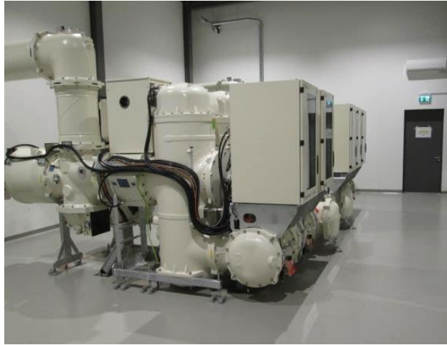
Fig 1.6 123kV C 4 F 7 N-CO 2 -O 2 gas mixture GIS substation [83]
