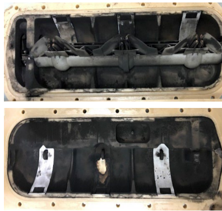
(a) Macro-morphology of the interior of the interrupter after disconnection
