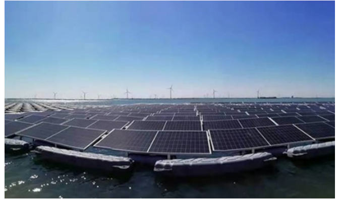
Figure 1.6 —Floating project developed by Huaneng Power International© in China's Shandong province, the installed capacity reaches 320 MWp
