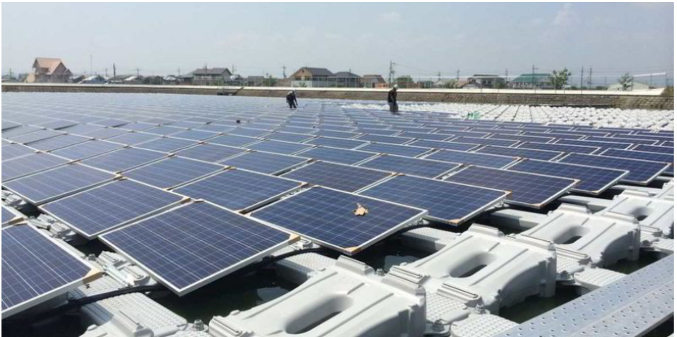
Figure 1.4 —An 850 kWp floating powerplant in Hyogo, Japan, based on the Ciel et Terre© technology.
