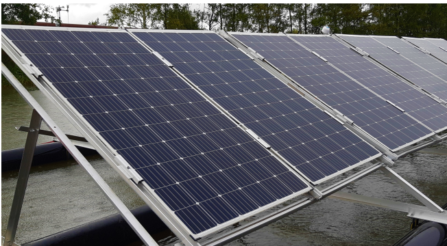
Figure 15 —Prototype of floating solar array installed in Belgium by EDF.
